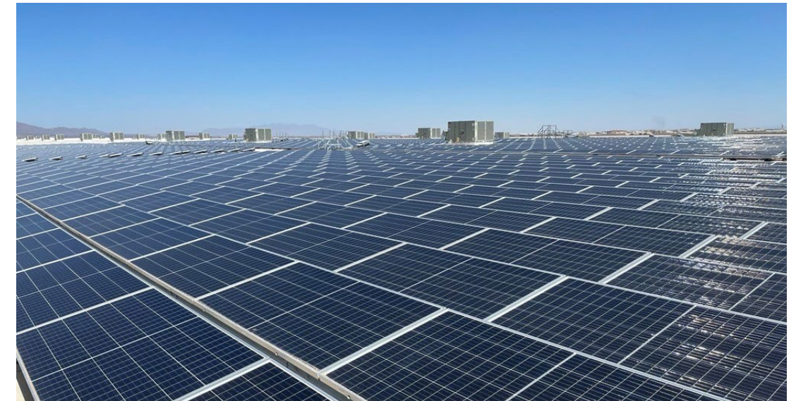
Rooftop solar panels at TJX's distribution center in El Paso, TX, became operational in Fiscal 2026
